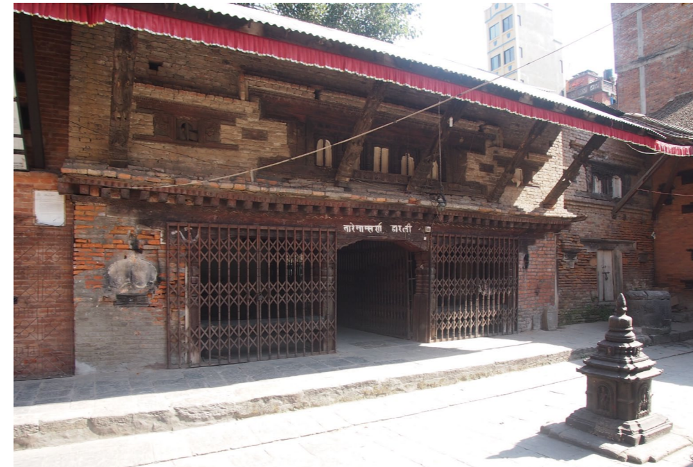
East wing, courtyard facade, existing conditions | 2012 Similarly to the east facade most brick work requires extensive repairs and replacement of material. The steel shutters will be removed and the timber elements of the open arcade ( dalan ) cleaned and restored.
