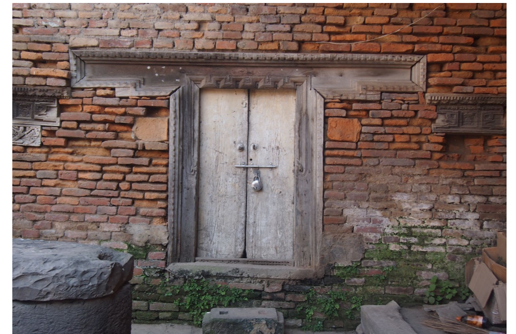
East wing, courtyard facade, existing conditions | 2012 A typical example of how rising damp has destroyed both the wall fabric as well as the lower parts of this historic door.
