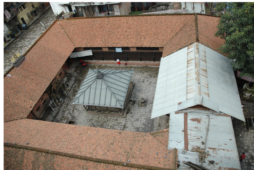
Itumbaha monastery | Sep 11, 2006 Following a three-year construction period 80% of the monastery was restored with funds from the German Foreign Office, the World Monuments Fund and the monastery's own contributions.
