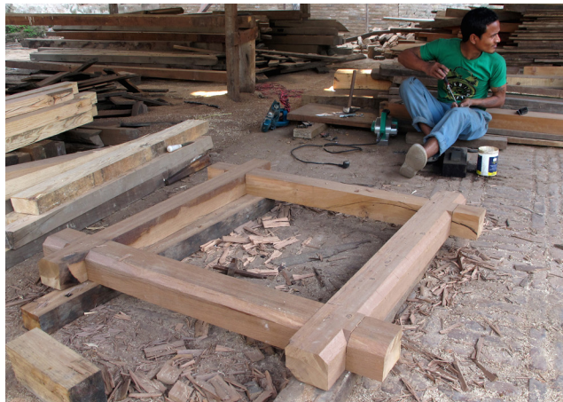
Reconstruction of timber collar | April 24, 2014 Carpenters fabricated a new timber collar using sal wood. The four timber elements were half-lapped to form a ring anchor.
