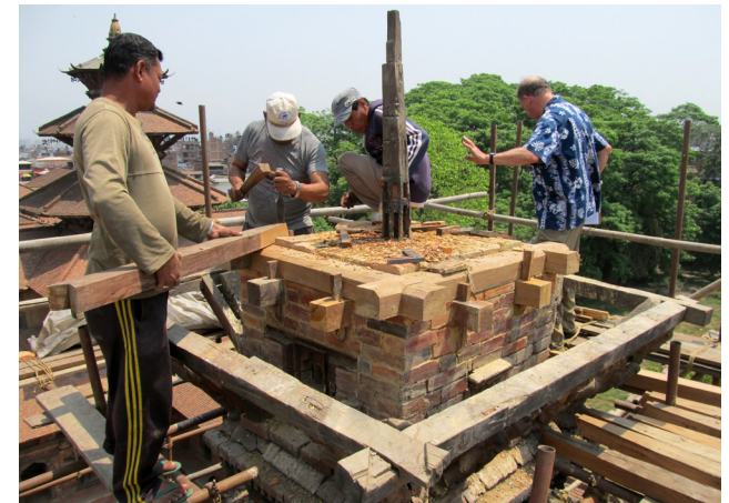
Fixing of rafters | April 27, 2014 A new joint was created 1' above the existing joint to fix the rafters to the existing central timber post.
