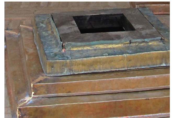
Reassembly of historic gilt sheeting | April 2014 The historic gilt sheet was installed over the new protective copper sheet. This original sheet was left intact since any restoration effort would risk damaging the gilt surface.
