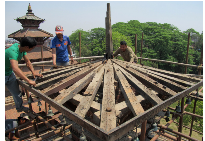
Inspection of existing rafters | April 22, 2014 All of the rafters were found to be unusable.
