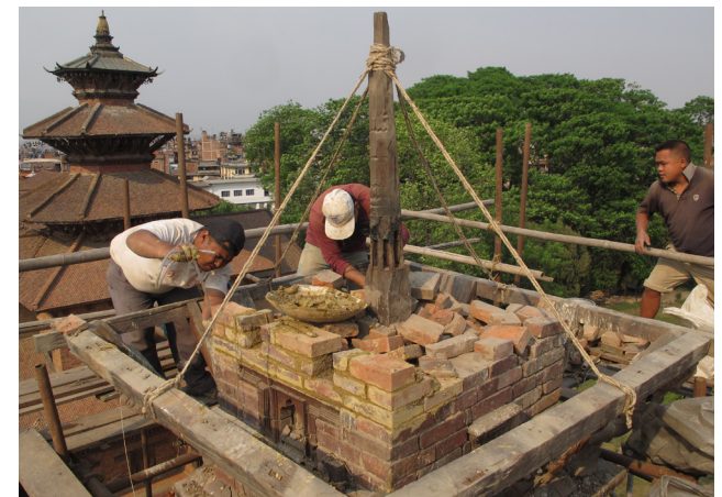
Reconstruction of masonry walls | April 25, 2014 The masonry wall was raised in preparation for the installation of the newly constructed hardwood collar ( see page 19 )
