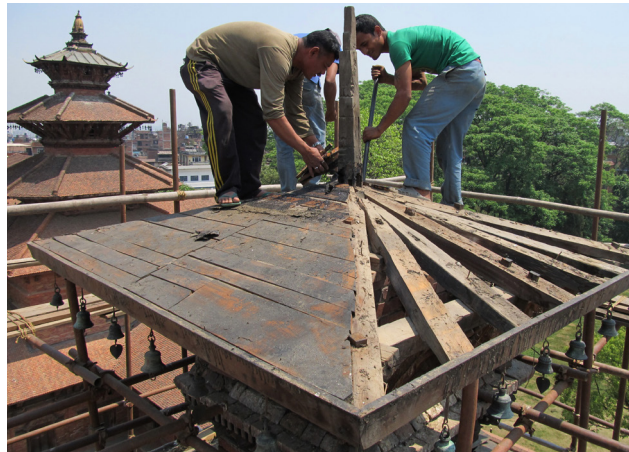
Removal of timber planking | April 22, 2014 The quality of the existing timber varied considerably: relatively new rafters were supported by rotten wall plates.
