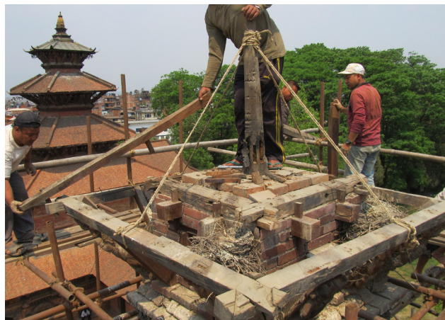
Removal of corner rafters and timber collar | April 24, 2014 The existing timber collar beams were found to be rotten.
