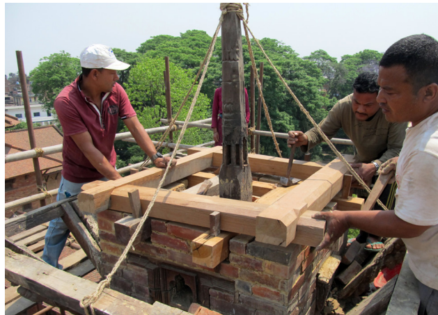
Installation of timber collar | April 27, 2014 The new timber collar was installed on top of the raised masonry on four cross pieces, optimizing the bond of the timber structure to the masonry.
