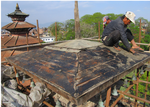
Removal of existing roof cover | April 18, 2014 The removal of the roof cover revealed heavily damaged timber planking.
