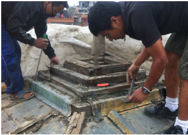
Removal of historic gilt sheeting | March 2014 The gilt sheeting was found to be extensively damaged with several holes allowing water to enter the timber structure.
