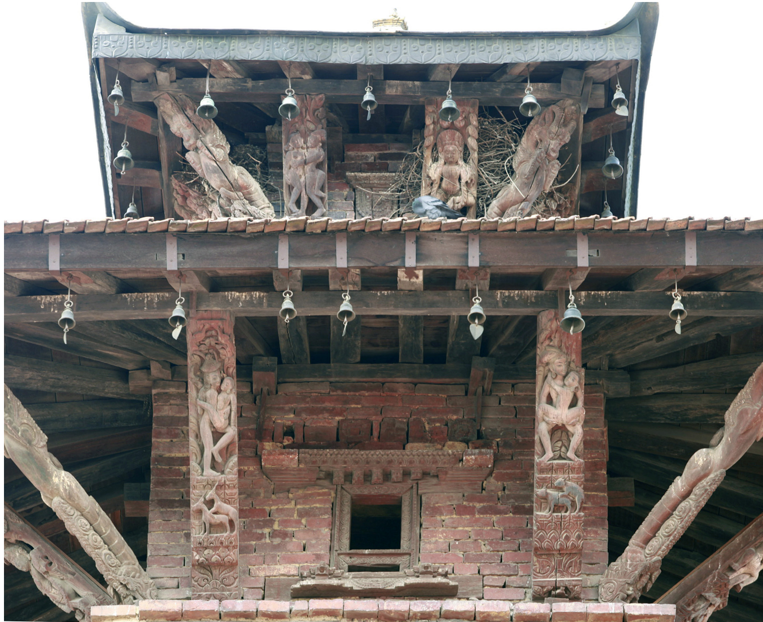
Second and third tiers | May 2013 This photograph shows the condition of the struts, rafters, and purlins of the second tier. Some of the struts depict Tantric divinities, while others feature various manifestations of Bhairabs and Matrikas. The 6 plain struts dating to 1994 were left intact.
