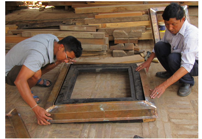
Sealing with protective copper sheet | April 2014 This protective copper sheet will prevent water infiltration into the timber structure.
