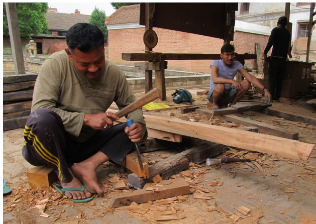
Fabrication of new rafters | April 28, 2014 New rafters were fabricated by carpenters with reference to the new roof design using both sal wood and pine.
