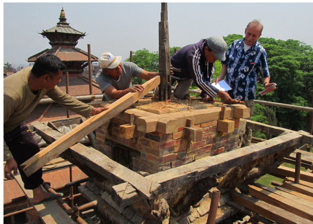
Fixing of central rafters | April 28, 2014 The new rafters were joined to the existing central timber armature.
