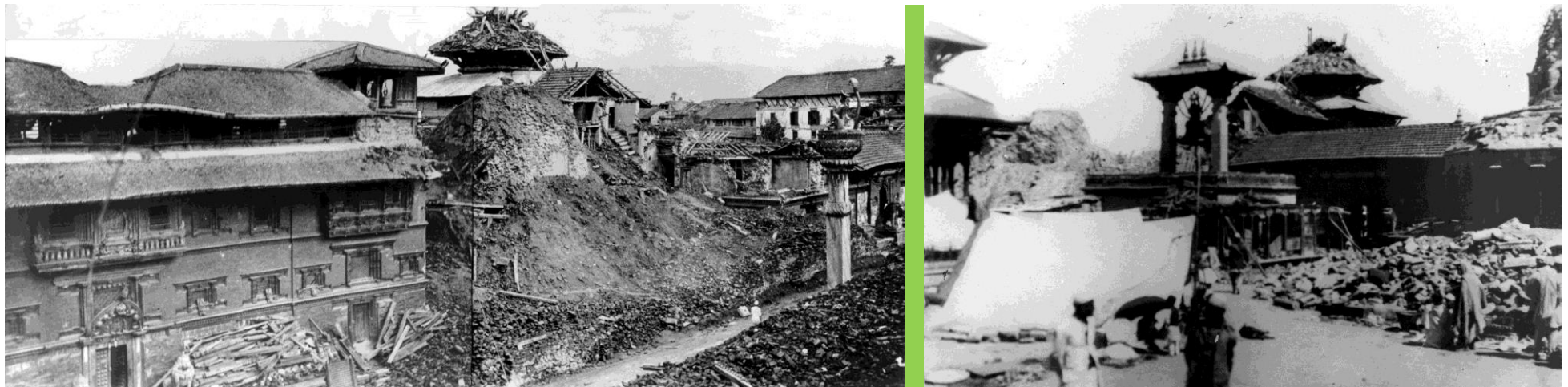
Damage from the 1934 Earthquake. Upper two levels of roof were completely collapsed in Taleju and adjacent wing on west lost more than half.
