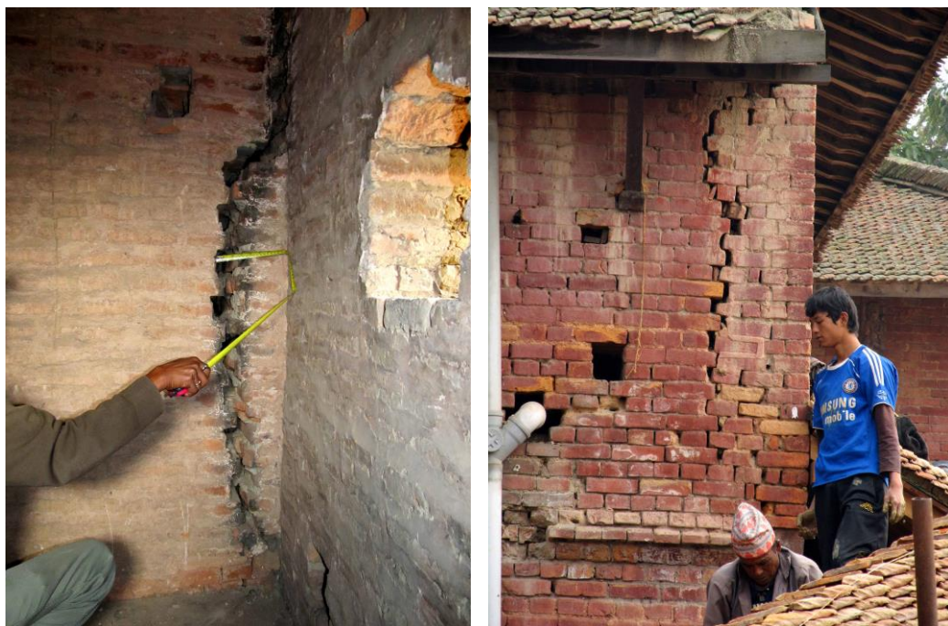
During the small September 2011 earthquake, the building performed comparatively well, although many of the already existing cracks widened.
