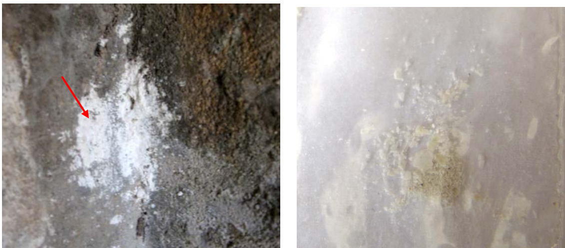
Figure 12: Location of Sample A3 (left) from the interior of the Bhandarkhal Tank pavilion and detail of sample (right).
