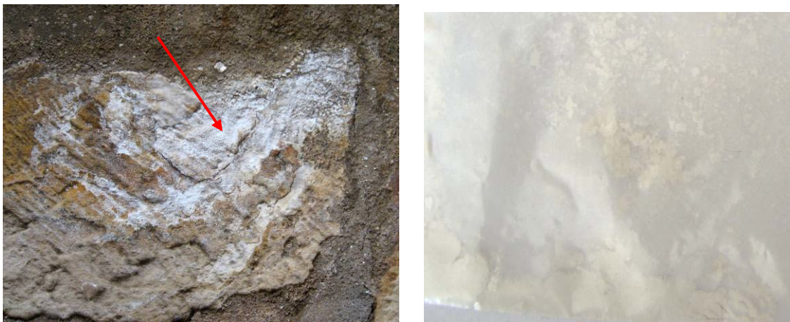
Figure 11: Location of Sample A2 (left) from the interior of the Bhandarkhal Tank pavilion and detail of sample (right).
