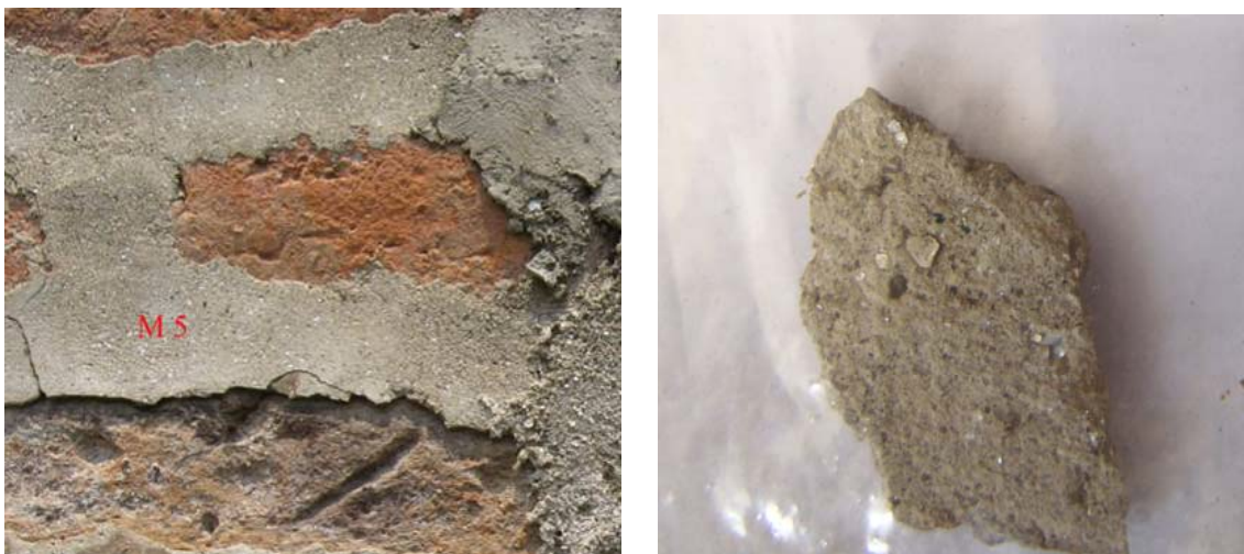
Figure 14: Location of Sample M5 (left) from the north wall of the Bhandarkhal Tank just below the pavilion and detail of sample (right).
