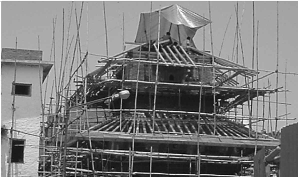
above: The ground floor arcade was built on reconstructed floor stepped plinth. The brickwork on the original plinth was in bad condition thus it had to be replaced. below: Rafters being installed for the two lower roofs.
