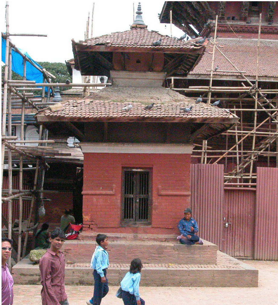
left: Lakshmi Narayan Temple, 2004. The original configuration of the temple was completely lost. When the Trust started its documentation, the roof structure was in a dilapidated state. The rafters were of inappropriate length and 50% of the roof tiles were lost, thus, allowing the rainwater to penetrate into the structure. The cement plaster had damaged exposing the corroded brick work. Photo by: Lumanti Joshi, August 2004.
