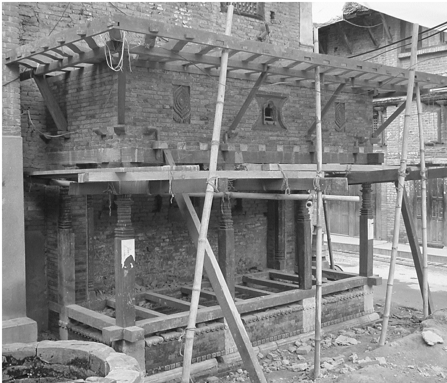
7. The upper wall above the beam built with newly carved elements in their positions.
