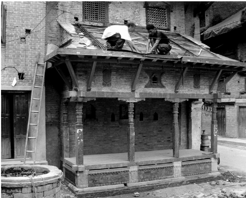
10. Waterproofing membrane being laid between the planks and the mud bed for tiles.
