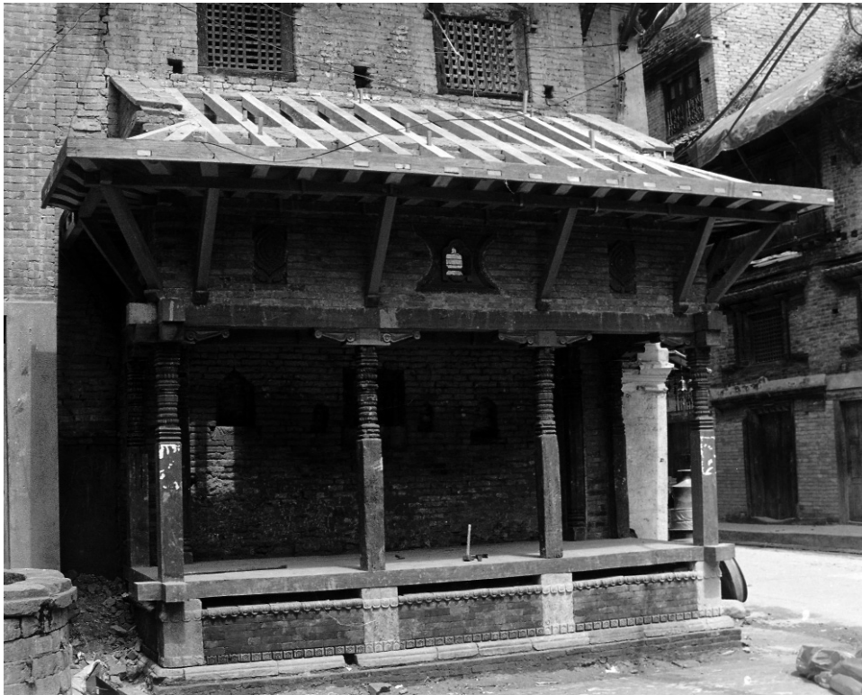
9. Rafters are installed with reference to the traces of a roof line on the wall of adjoining house.
