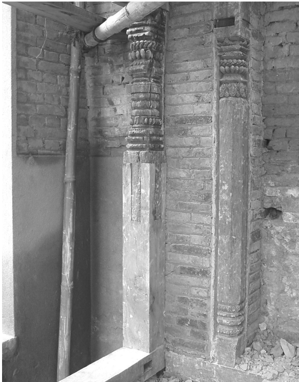
6. Newly carved columns being erected next to the old one. The base of one of the originals was retrofitted with new timber to provide stability to the structure.
