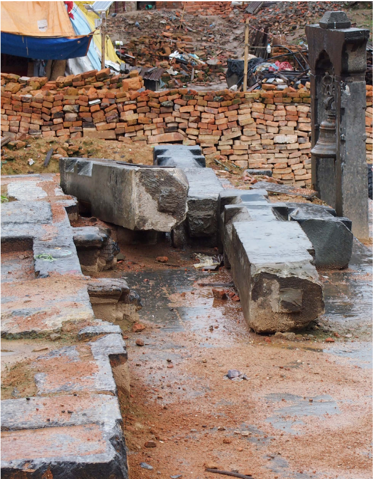
Four of the 20 stone pillars which supported the arcade Note the very shallow tenons which did not provide sufficient positive bond to the structure below. Photograph Thomas Schrom | July 20, 2015
