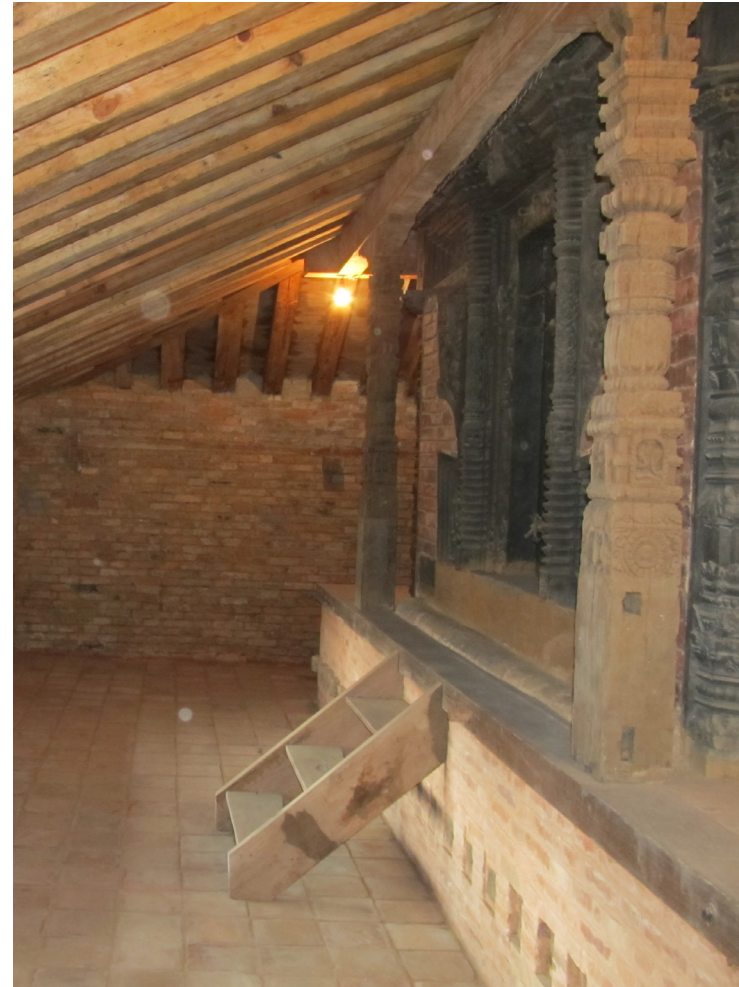
South side of the sanctum after restoration | October 2012 Note the improved condition of the masonry plinth, which was completely re-built. A new timber frame on the outer edge acts as a brace against seismic movement. The beam supporting the rafters was moved as close to the sanctum's structure as possible, and was connected to the sanctum with steel bolts and straps.
