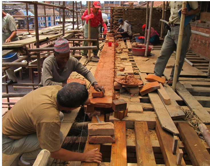
left: Continued re-building of the east-facing wall. Note the proper integration of the timber window frame into the masonry.
