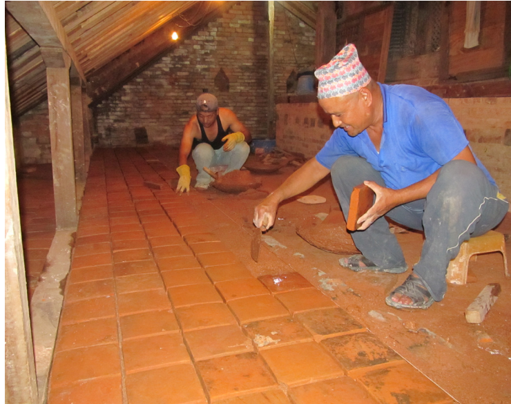
far left: Brick soling being laid in the north west corner of the third level.
