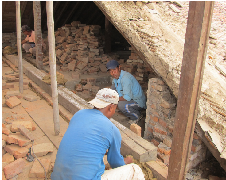
far left: The east-facing wall was beyond in-situ repair after it was badly damaged by the 2011 earthquake. Here the wall is being dismantled.
