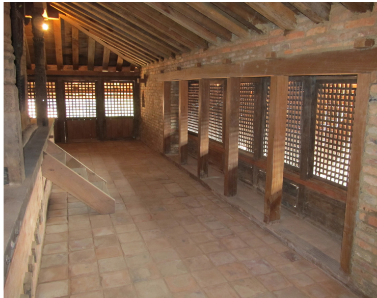
far left: Telia floor tile being installed over the soling on the east side of the third level.
