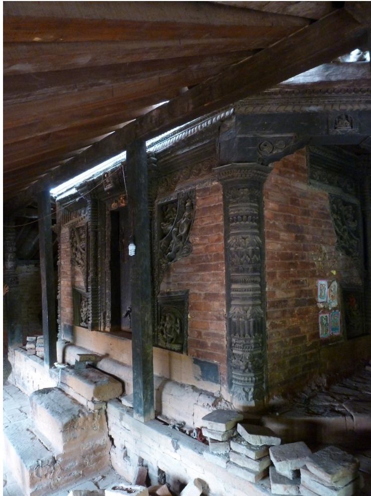
South side of the sanctum before restoration | April 2012 Note the strip of light along the top of the sanctum's cornice. This light is entering the third level via the large gap between the roof structure and the sanctum's walls. The chief focus of this seismic upgrade was to improve the structural connection between the inner sanctum's masonry structure and the surrounding roof. Also note the poor condition of the plinth.
