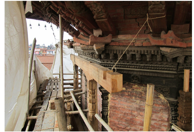
Placement of crossbeam atop historic columns | August 2012 As was planned in the original seismic report, the new system of columns and beams was installed around the inner sanctum. Historic columns were used, and were strategically placed before each corner column of the sanctum.
