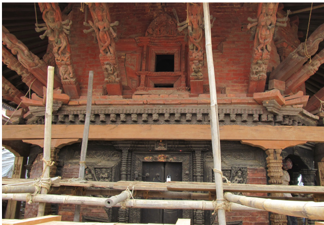
Frontal view of timber support system | August 2012 This photo shows the newly installed columns, capitals, and cross beam along the sanctum's south-facing side.
