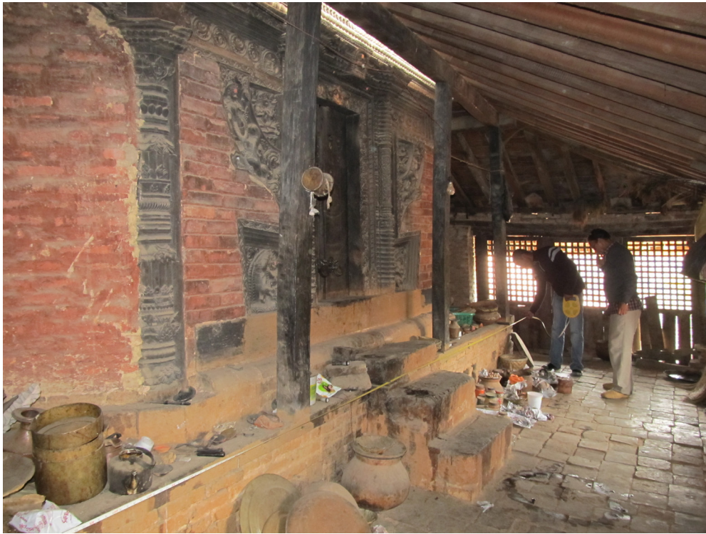
South side of the sanctum before restoration | April 2012 Note the sagging of the rafters and the make-shift columns and beam supporting the roof, part of an inadequate recent intervention.
