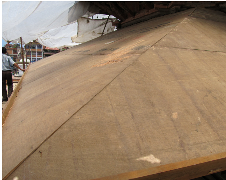
far left: As was done with the floor, plyboard is installed over the roof planking to create a rigid diaphragm.
