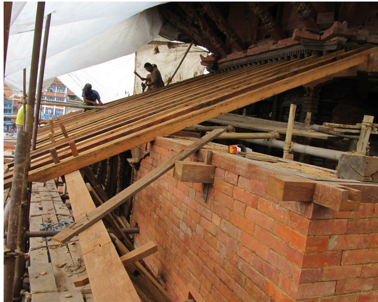
left: The south-facing wall being rebuilt with new brick in an interlocking arrangement to ensure both the south and east walls are sufficiently tied together.
