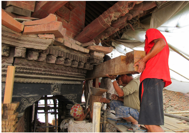
Installation of new timber support system | August 2012 One of the new horizontal beams which runs along the face of the carved cornice is carefully moved to its position. This beam will serve as the force-fit connection between the roof and the inner sanctum. This will securely connect the roof structure to the inner sanctum core.
