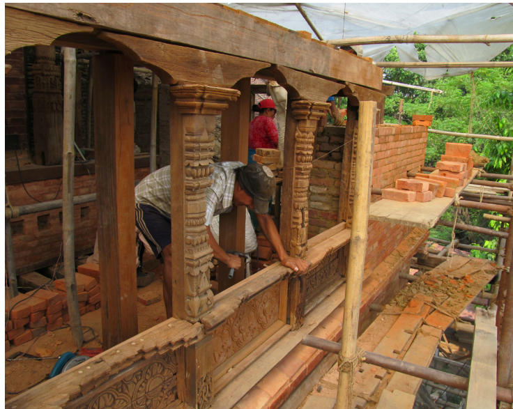
left: The east-facing wall being built around the new window frame. The timber frame was properly integrated into the surrounding masonry.
