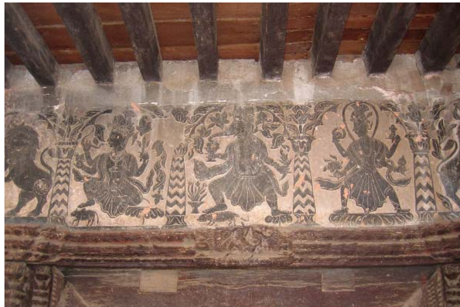
Sgraffito frieze above the main entry to the Court Building A rare surviving example of sgraffito offers the opportunity to develop conservation and restoration methods for this decorative technique employed on early 19th century buildings.
