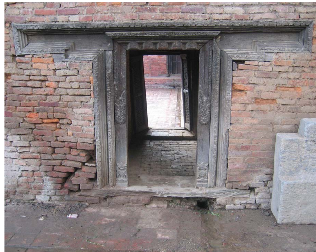
far left and left: Two doors on the Garden facade Until recently, the back courtyard was covered with debris which caused irreversible damage to the doors. A large variety of bricks found in this wall suggests that this part of the building has been repaired in patches until very recently. Some historic daci-apa bricks can be found only in isolated locations. They are certainly not found in situ but were reused from demolished walls. Photograph, May, 2006
