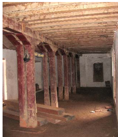
Main hall on the ground floor This space could be adapted for exhibition or retail space. Photograph, May, 2006
