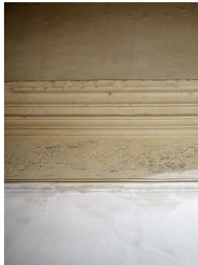
far left: North Wing - storage room on first floor level Most the North Wing's rooms are used for the storage of broken furniture.
