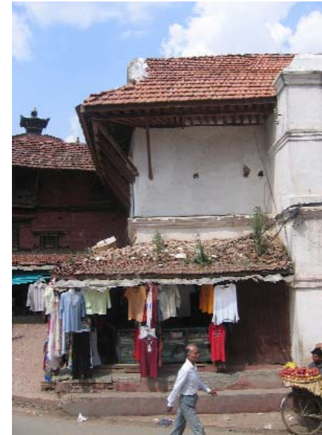
South-west corner of the Court Building Commercial encroachment.
