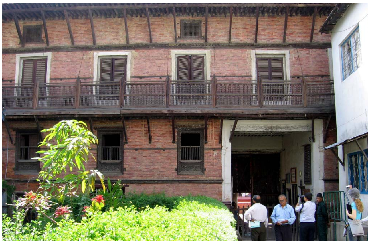
North wing - east facade This part of the building retains most of its original form. Repairs of doors, windows, balcony, and roof were carried out with the support of the German funded Urban Development through Local Efforts Programme in 1995. Photograph, May, 2006
