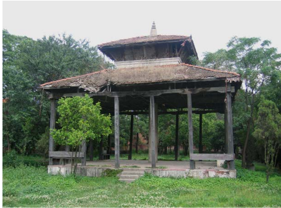
Object #07: Concrete and timber pavilion with collapsing roof, (built for King Birendra's coronation)
