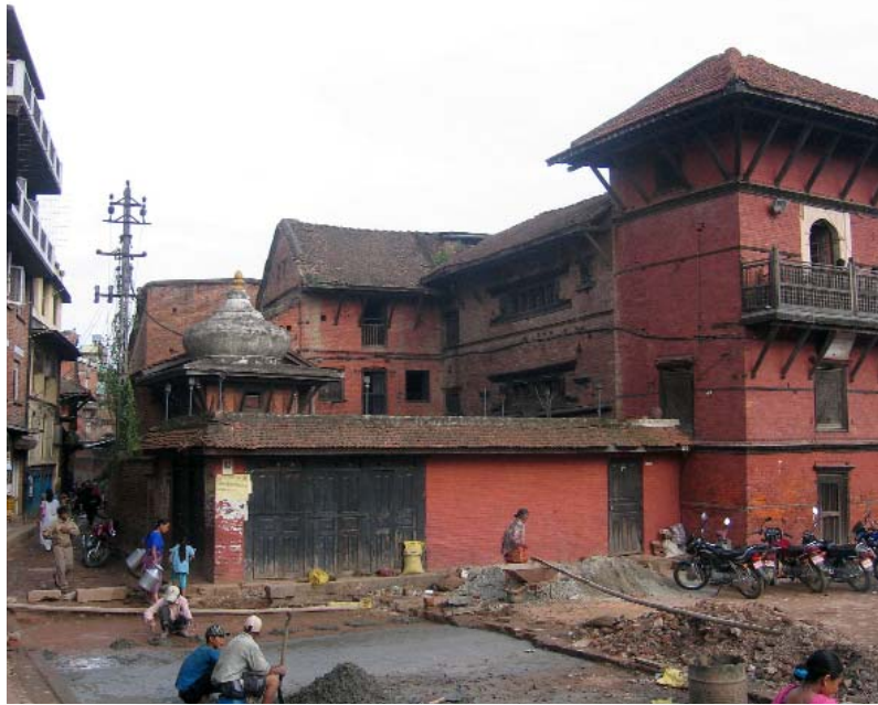
Object #01: one-story structures built illegally around the small Shiva shrine. After demolition there will be public access to the temple and the 17th century agam building.
