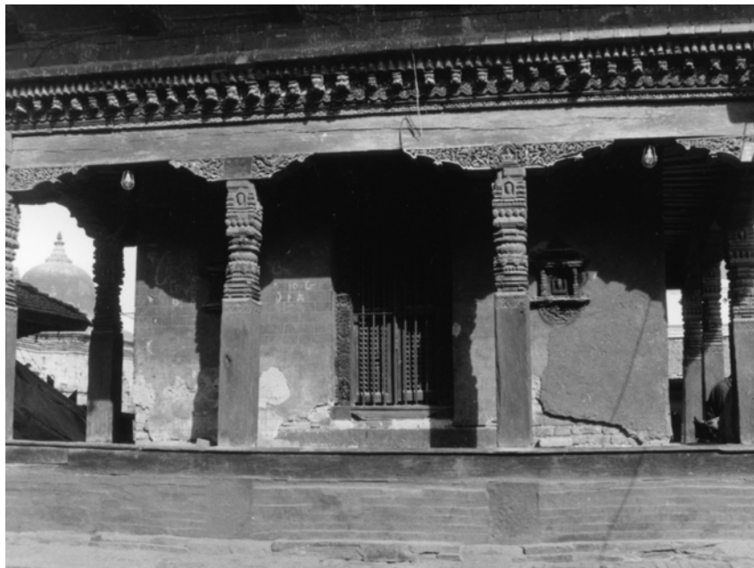
above left: The dilapidated condition of the roof structure on the east facade prior to the restoration. Photo: Rohit Ranjitkar, April 2003.
