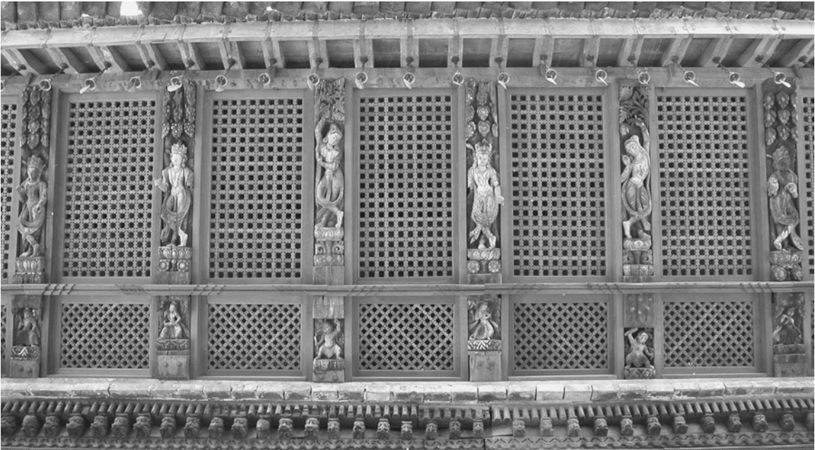
above: Carvers fabricating the details of the lattice window for the first floor level with reference to the drawings and photographs provided to them. Photo: Heike Pfund, November 2003.
