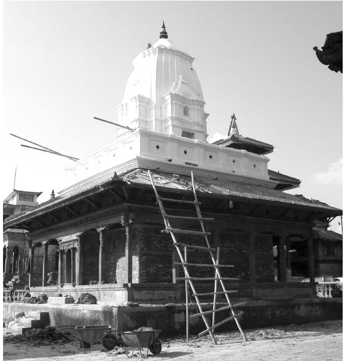
top: Battens being fixed on the roof structure to hold the mud in its position. Water proofing membrane was introduced between the planking and mud bed. Traditional roof tiles ( jhingati ) were laid on the mud bed. Photo by: Raju Roka, KVPT, October 2005. right: Final stage of completion. Photo by: Raju Roka, KVPT, October 2005.
