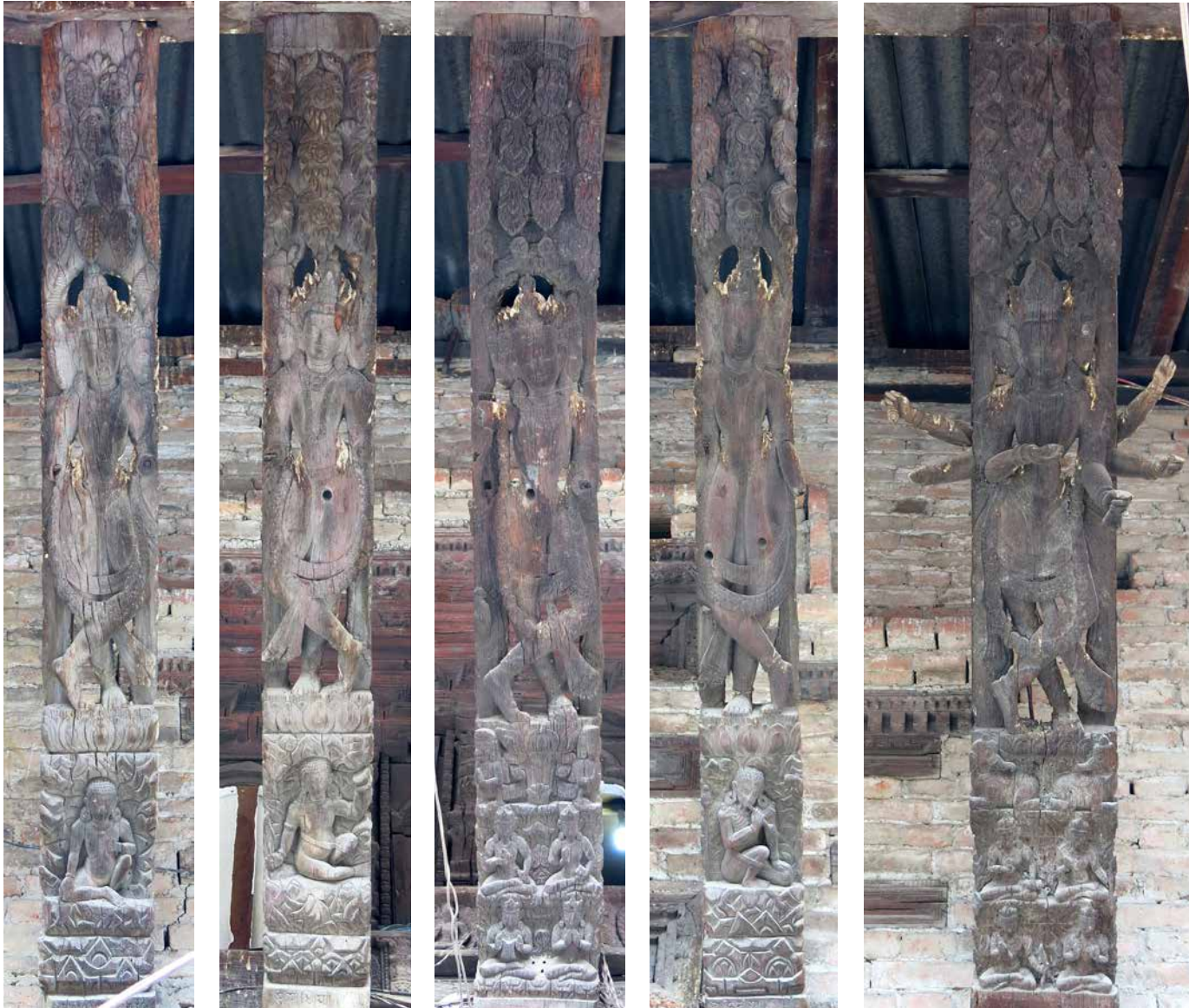
Roof Struts of Itumbaha | June 2014 Roof Struts of east wing courtyard facade in damaged poor condition due to rain water leakage from roof.
