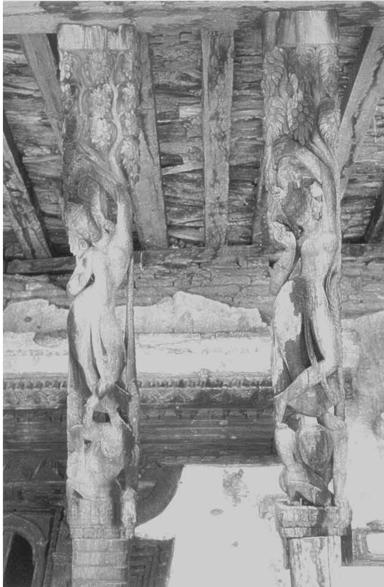
Roof Struts of Itumbaha | August 1999 Struts with poor condition due to rain water leakage from roof.
