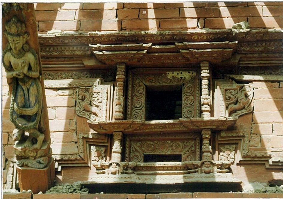
UPPER BASE STORY WINDOW ABOVE ENTRANCE, WEST ELEVATION. FEBRUARY, 1992. SEE DISCUSSION OF FRAME ELEMENTS PAGE 13.
