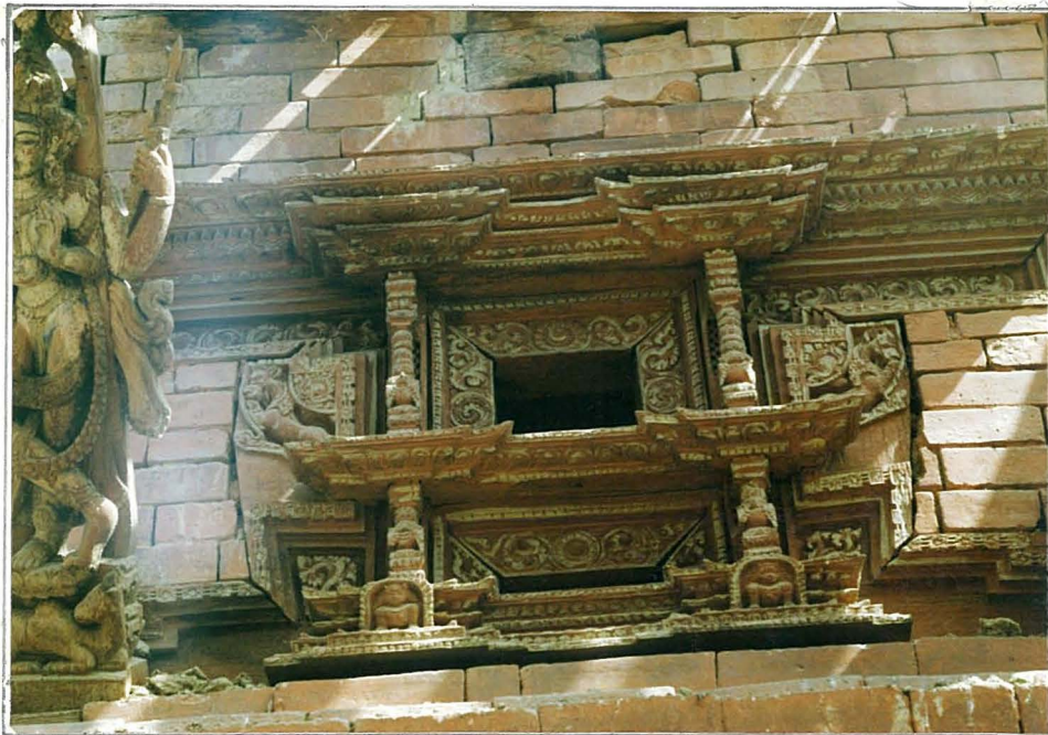
ABOVE: INTACT WALL SURFACE OF UPPER STORY AT NORTHEAST CORNER. BELOW: UPPER BASE STORY WINDOW, SOUTH ELEVATION. JANUARY, 1992.
