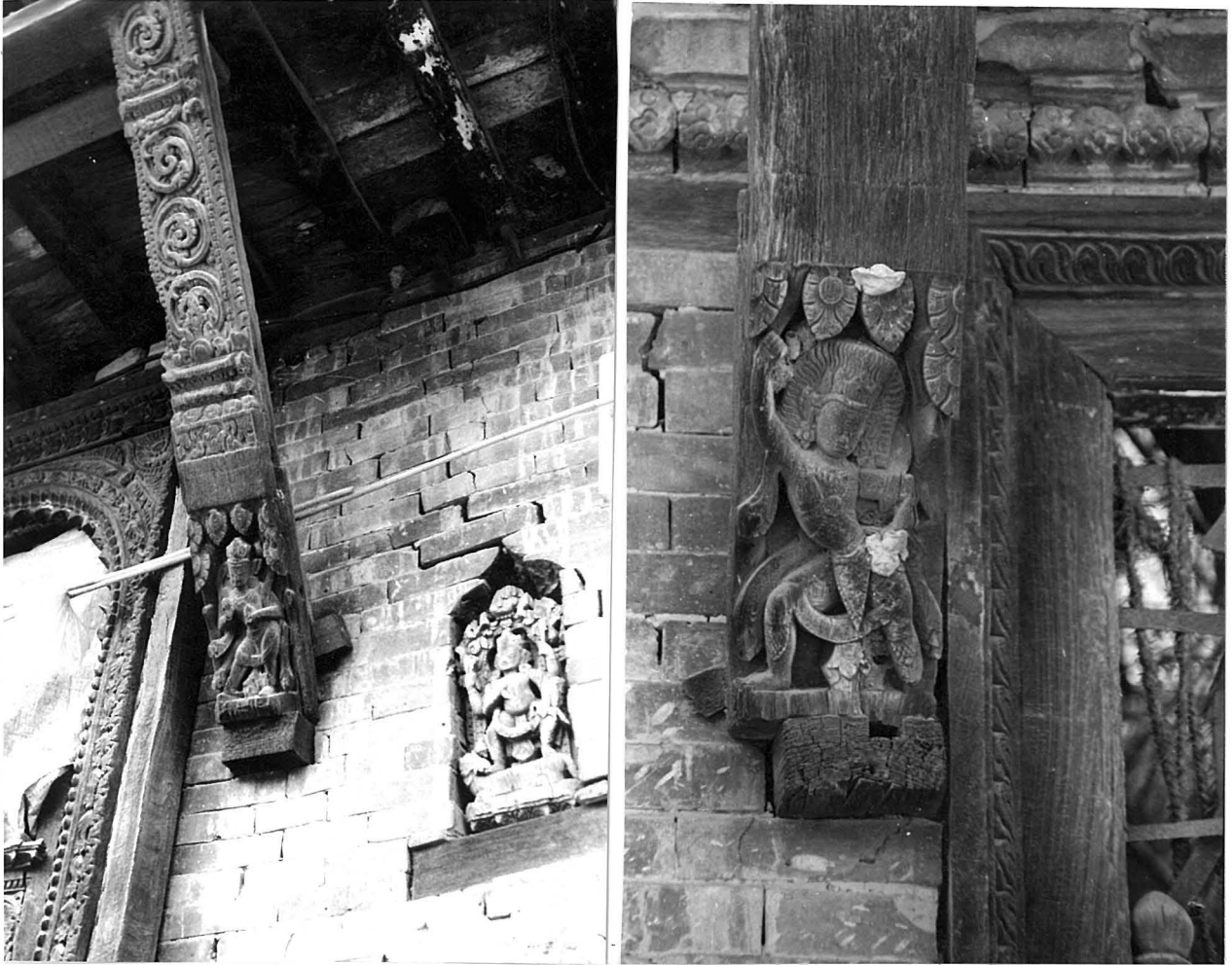
Roof struts (Newari: tunah ). Five existing carved struts come from a leaning bay window (Newari: san jhyah ) as demonstrated by tenons visible on the sides of each piece and the format, which would be unusual for a typical roof strut. The struts are divided into two registers with varying figures below and repetitive wave motifs above. Struts numbered left to right 1-5). Opposite upper left: strut#1 with Bhairav figure; upper right: strut #2 another pose of Bhairav; opposite lower left: strut # 3 Visnu. This page left: strut #4 Siva and right #5, Siva (?).
