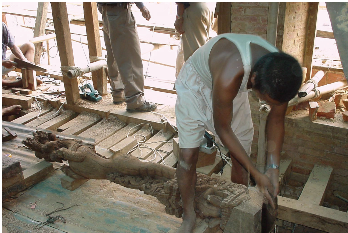
A carpenter shaping the timber for replacing rotten base area of the historic strut. Photo: Rohit Ranjitkar, August 2002.
