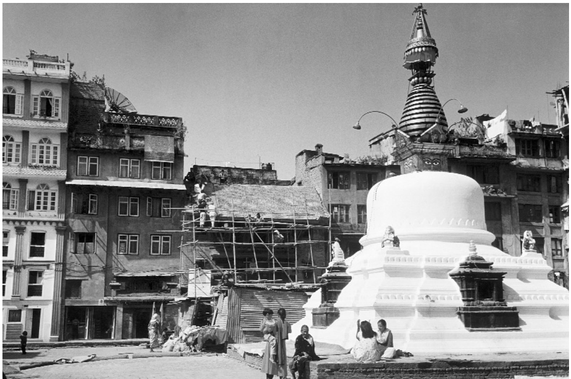
Jhingati (historical roof tiles) being laid over the mud bed. Photo: Heike Pfund, October 2002.
