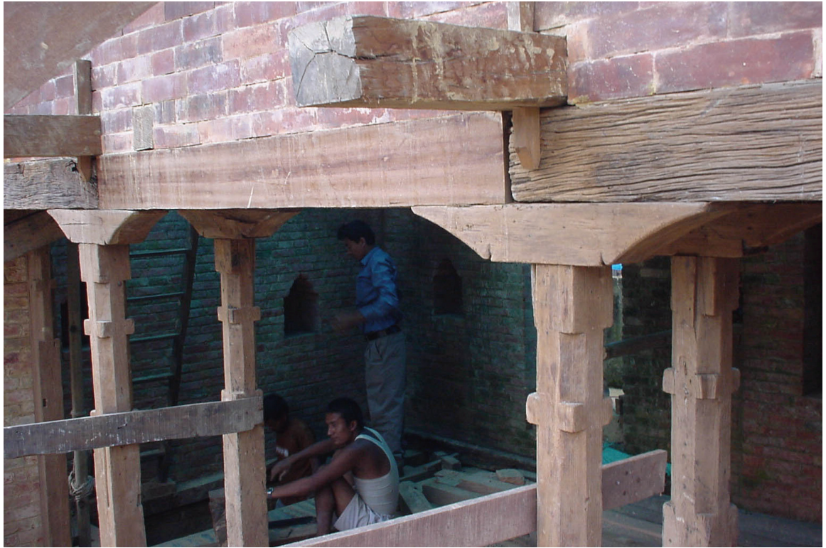
The historic pillars, capitals and beams were reinstalled after cleaning. New beams added to replace the deteriorated portion. Photo: Rohit Ranjitkar, August 2002.
