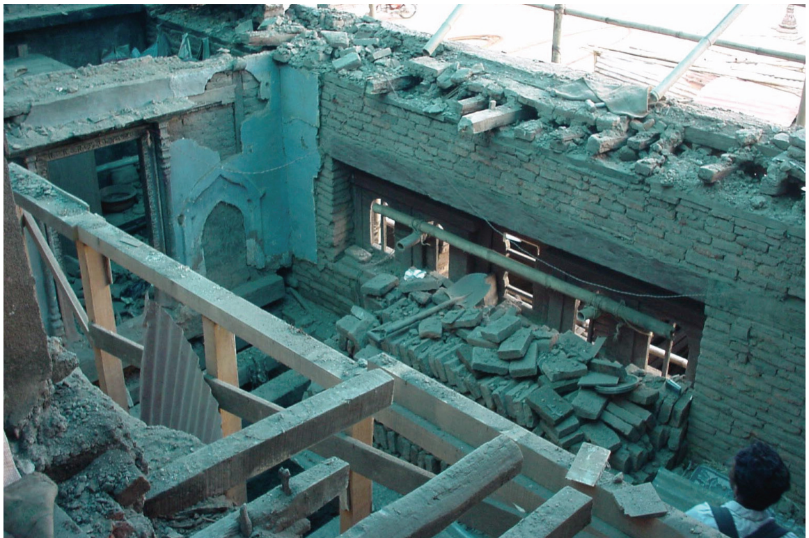
Joist at attic and 2nd floor level dismantled to replace with historic size timber and spacing. Photo: Raju Roka, May 2002.
