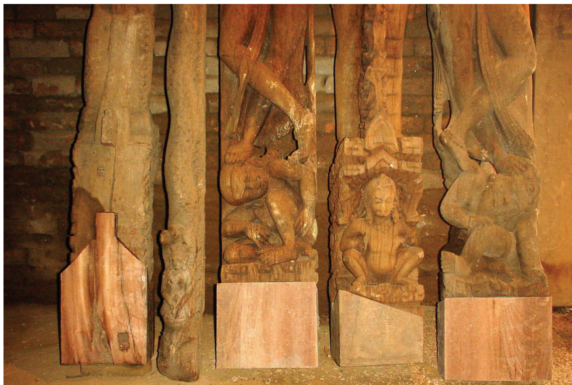
The 13th c. historical roof struts were repaired by replacing decayed portion of the struts. Photo: Raju Roka, August 2002.
