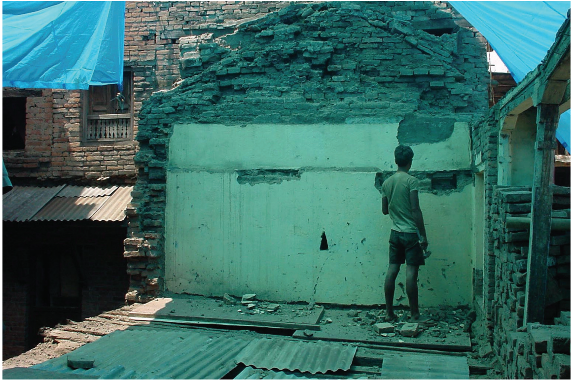
Later added zinc sheet roof and 2nd floor level brick wall dismantled in order to rebuild in historic figure with traditional material. Photo: Raju Roka, May 2002.
