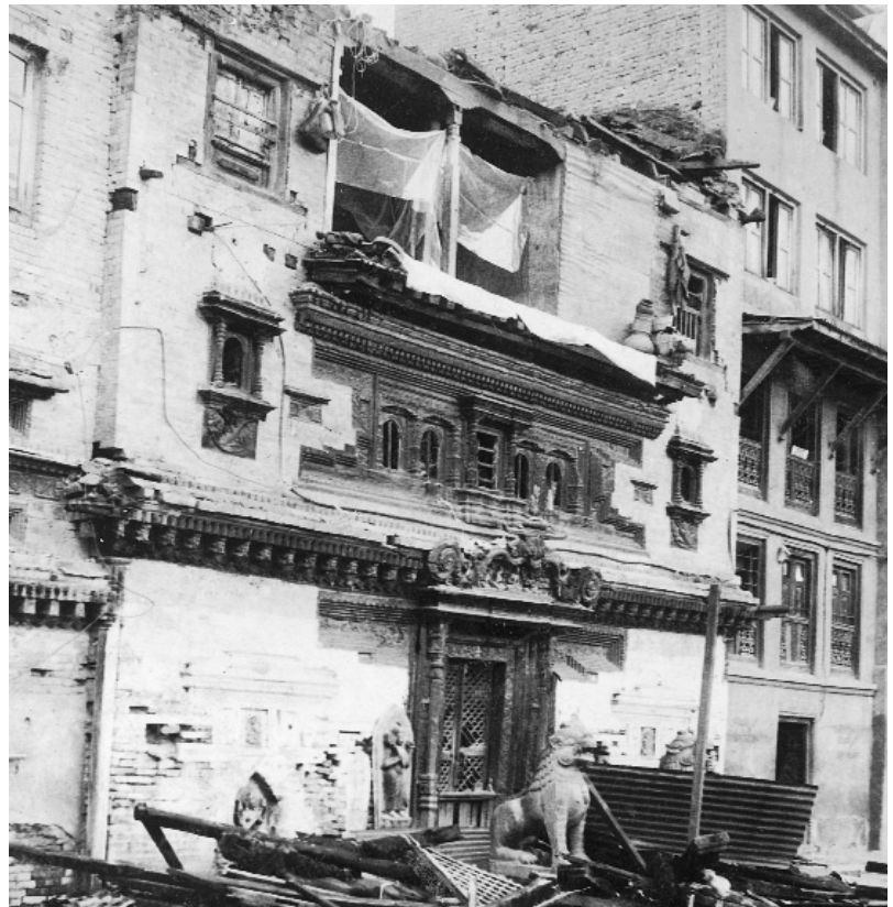
A picture showing complete collapse of roof in 1987.
