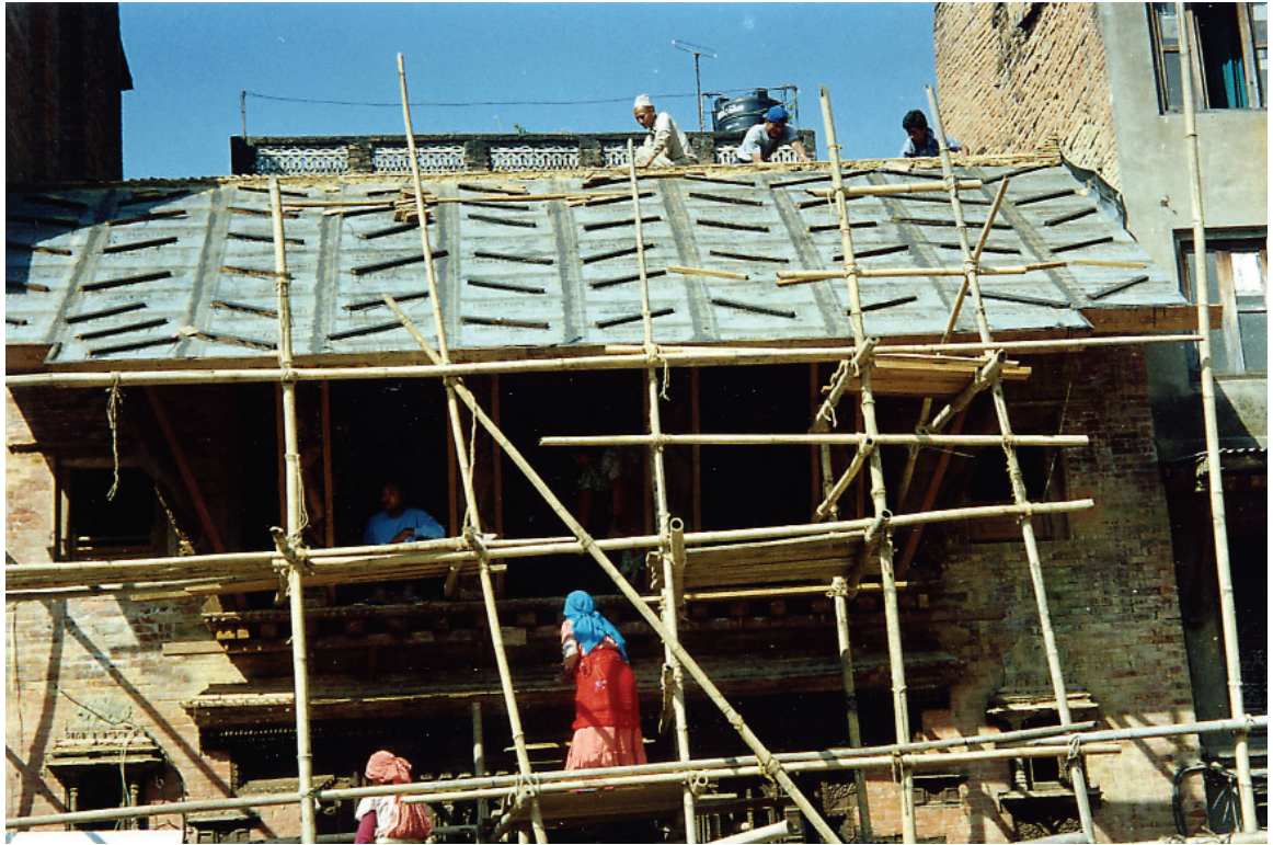
Roof water proofing membrane being laid over planking to prevent water penetration during the rainy season. Photo: Raju Roka, October 2002.
