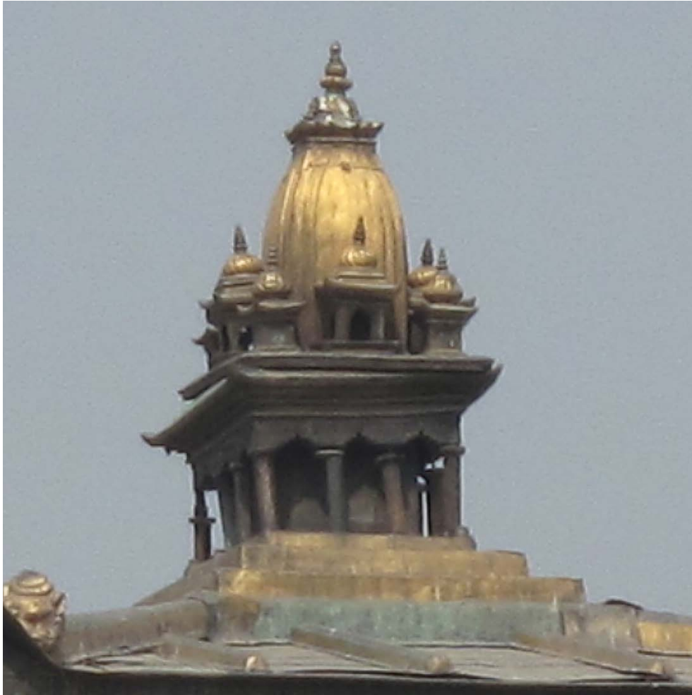
South Taleju Pinnacle view from the south | March 2013 This view shows the pinnacle's poor condition. Much of the gilding has worn off and separation of copper sheets can be observed.
