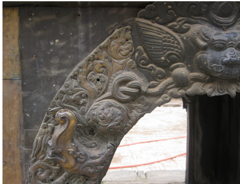
Detail of arch | Nov 2011 When the monument was repaired in the mid 20th century, replacement parts were not only poorly made but also not gilded, as is demonstrated by this detail. Here, the left part of the arch is original, while the center head is a later addition.
