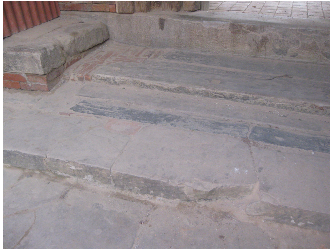
Brick filling and damaged stone | Nov. 2011
