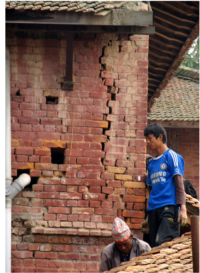
B: Detail of west-facing exterior facade crack | Nov. 2011
