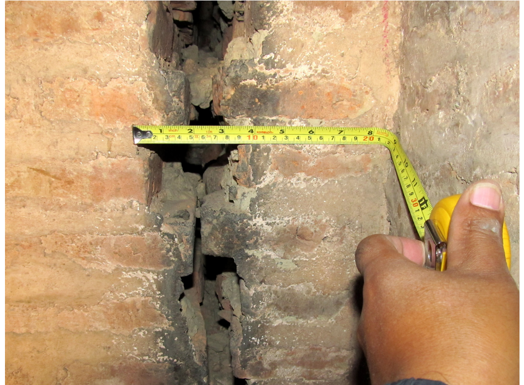
A: Detail of interior north wall crack | Nov. 2011
