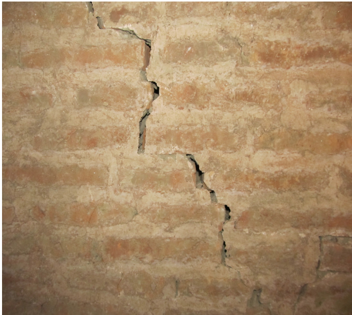
C: Detail of interior south wall crack | Nov. 2011 This detail shows the freshness and severity of the crack. Such a crack will be repaired by careful extraction of the affected and surrounding bricks, and replacement with traditional, high-fired “ma-apa” brick.
