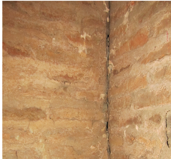
E: Cracking in southeast corner and fissure between walls | Nov. 2011 The southeast corner suffered some very minor cracks which are seen here. A small fissure occurred between the two walls, which are not properly joined and are therefore prone to break apart in the event of seismic movement.
