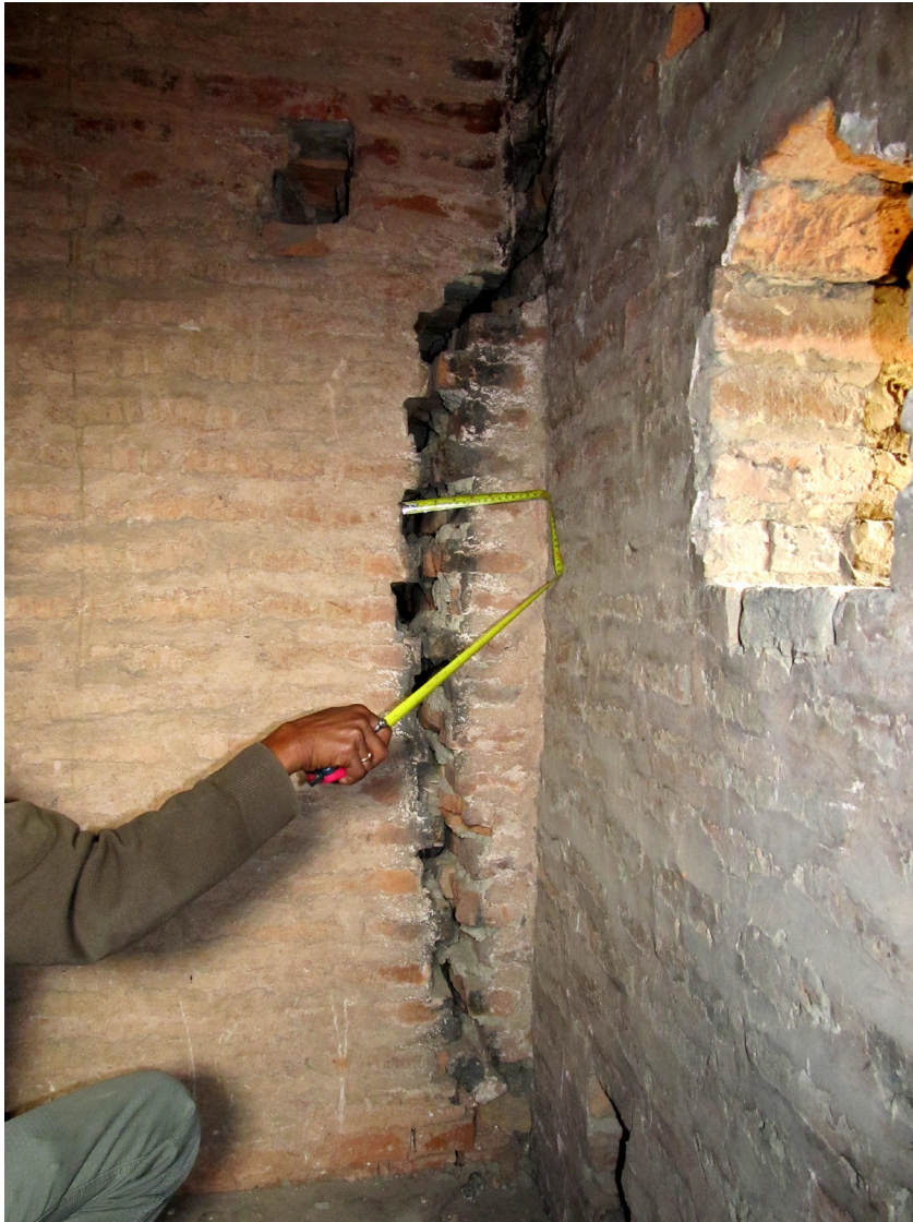
A: Crack on interior north wall | Nov. 2011
