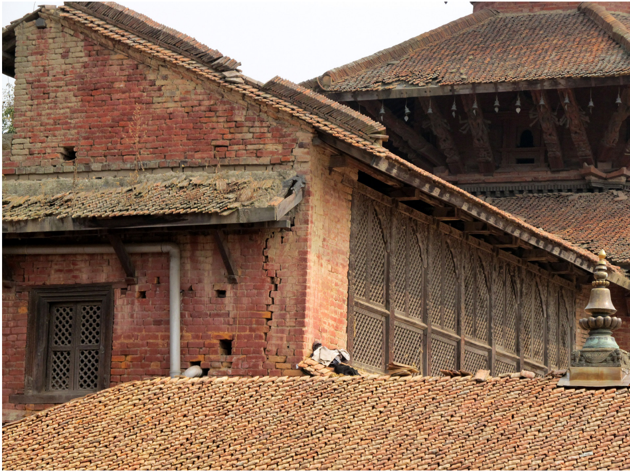
B: Crack on the west-facing exterior facade of Taleju | Nov. 2011
